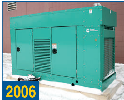
2006 CUMMINS G GHH - 5774586 EMERGENCY STAND-BY AC POWER GENERATOR
